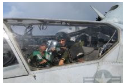
Sgt Eric Driz, left, and Cpl Diego Ascencio replace an environmental control unit in an AH1 Cobra helicopter.
